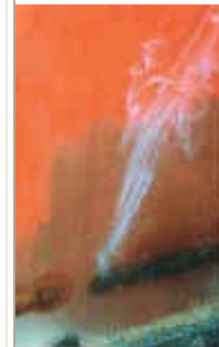
Smoke from burning paint along a line of weld being laid down on the other side of this steel plate.
